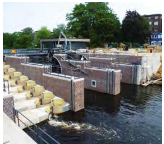
Fuhlsbüttel sluice with fish ladder
